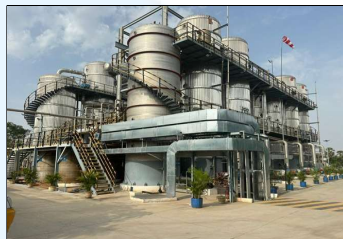
2 MLD Leachate Treatment Plant, Hyderabad, TS
